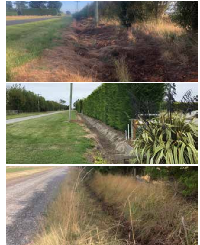
Powerlines, roads, and fences are often located close to drainage waterways, making bank reshaping and planting a challenge where required.
