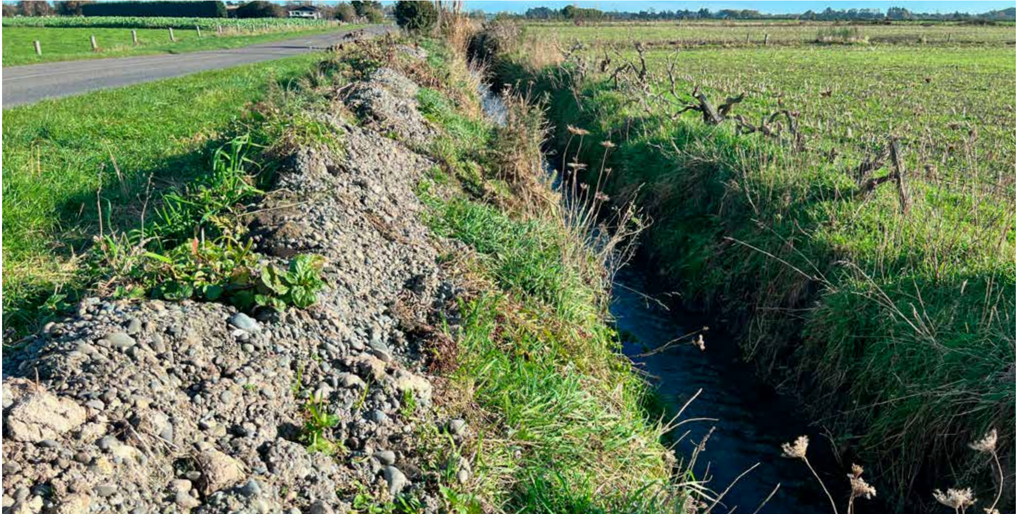
Spoil left alongside drainage channels can divert flood flows onto adjacent lower lying land or prevent floodwaters from readily re-entering the channel once overtopping has occurred.
