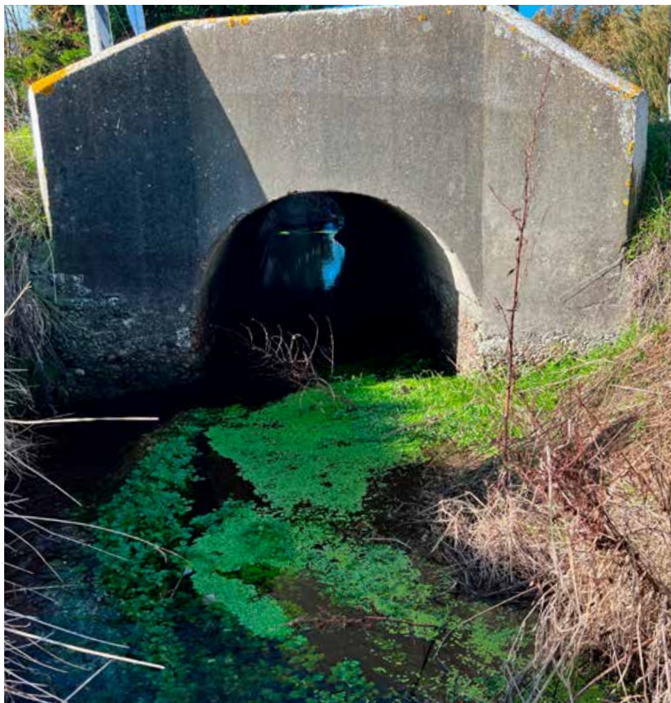
Example of an undersized culvert in the Leeston rated catchment.
